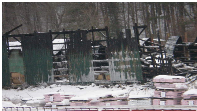
Building products storage fire
