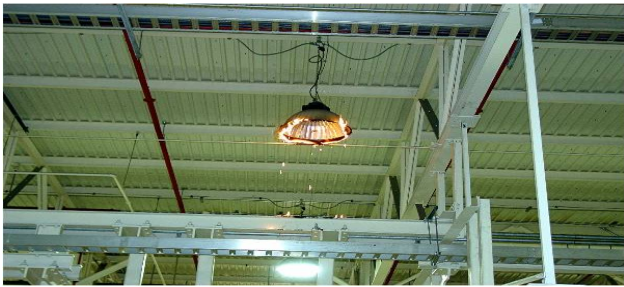
HID Lighting with cover beginning to burn. Photo compliments of ISO.
